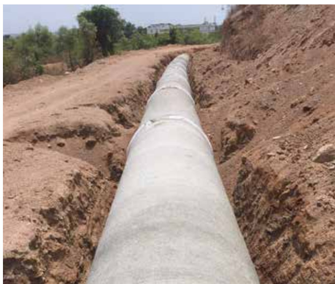
1500 mm dia PCC pipeline laying at Balkonda Water Supply Scheme in Telangana
