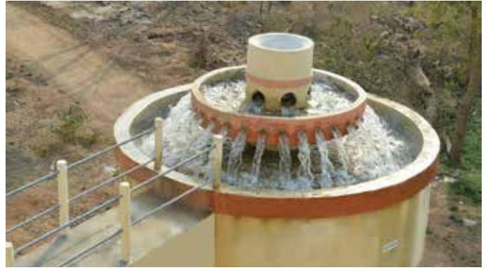
Aerator at Chhindwara Water Supply Scheme in Madhya Pradesh
