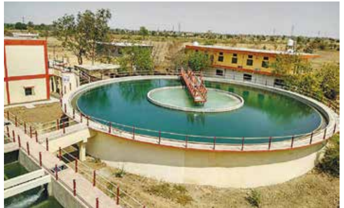
19.5 MLD Clariflocculator at Ganj Basoda Water Treatment Plant, in Madhya Pradesh
