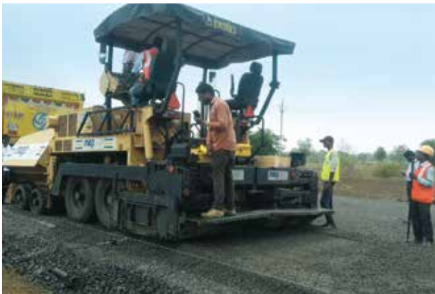
Dry Lean Concreting commencement in Nagpur Ring Road by using concrete batching plant having capacity of 120 cum per hour
