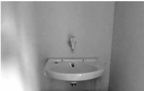
Piped water connection at 6 Anganwadi centres in Dahej, Gujarat.
