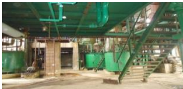
Sulphuric Acid Plant
