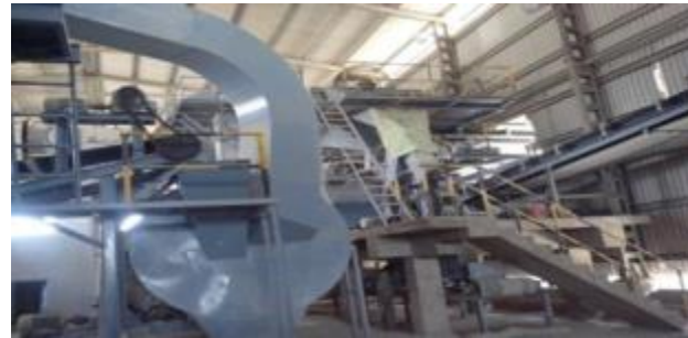
Unit 2– Granulation Plant
