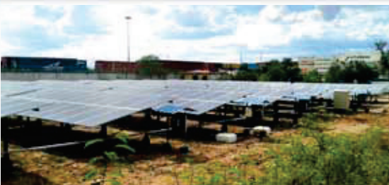
In 2016-17, 200 KWp of Solar Plant was installed at Manali, Chennai which is capable of generating 27000 units of power per month and offsetting around 300 tons of carbon dioxide each year. This plant will supply power to the Greases & Lubricants, Industrial Packaging and Leather Chemicals manufacturing units at Chennai.
