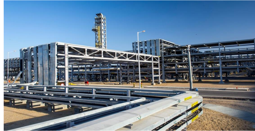
Rajasthan: Mangala Processing Terminal
