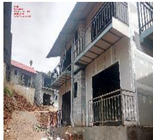
Resorts Partitions & Mezzanine Flooring
