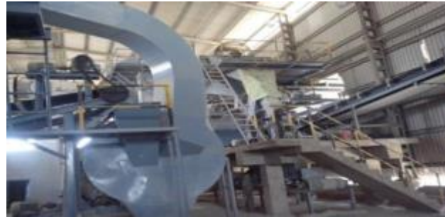
Unit 2 – SSP Granulation Plant
