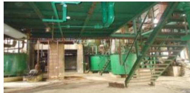
Sulphuric Acid Plant
