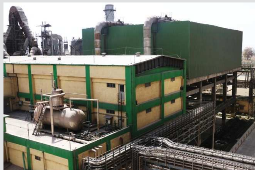
Waste Heat Recovery System
