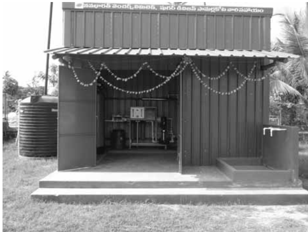
RO Plant at Sri Kumara Rama Bhimeswara Swamy Temple, Samalkot
