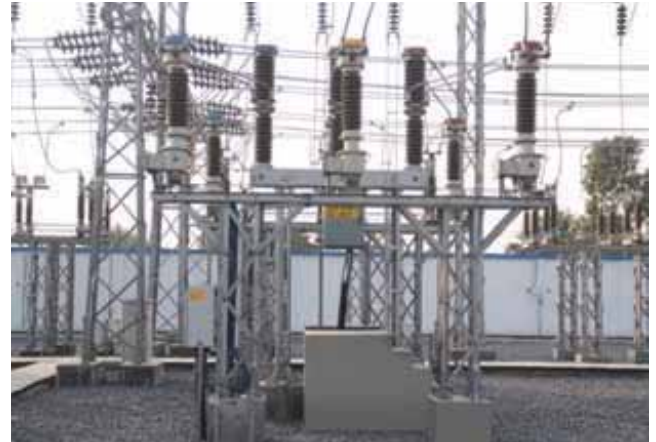
HT Electrical Systems for Tata Power Substations, New Delhi
