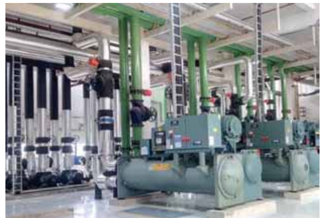
HVAC Systems for Mars International, Pune
