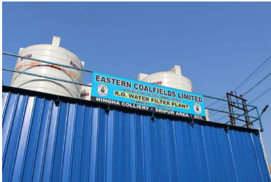
Fig. 36- R O Plant in ECL
