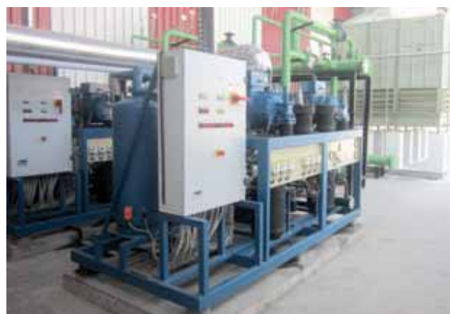
Refrigeration System for Hatson Agro Products, Chennai
