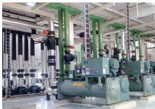
HVAC Systems for Mars International, Pune
