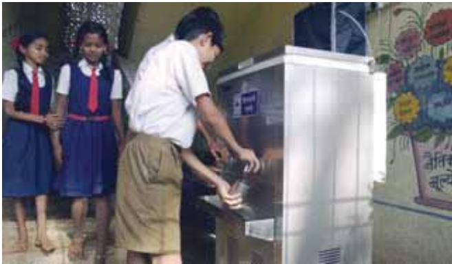
Drinking water station installed at a school in Wada
