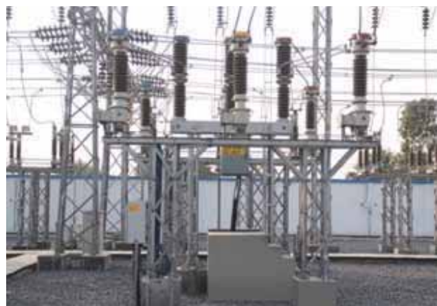
HT Electrical Systems for Tata Power Substations, New Delhi
