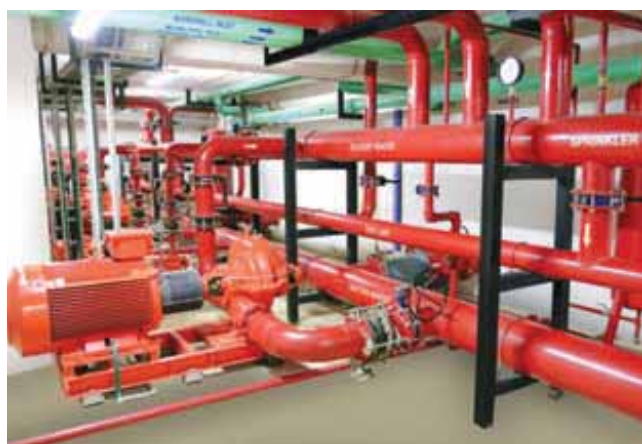
Mechanical, Electrical and Plumbing Systems for VR Mall, Chennai
