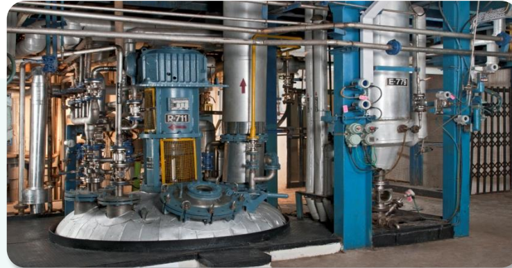
Agro Chemical Plant - Panoli
