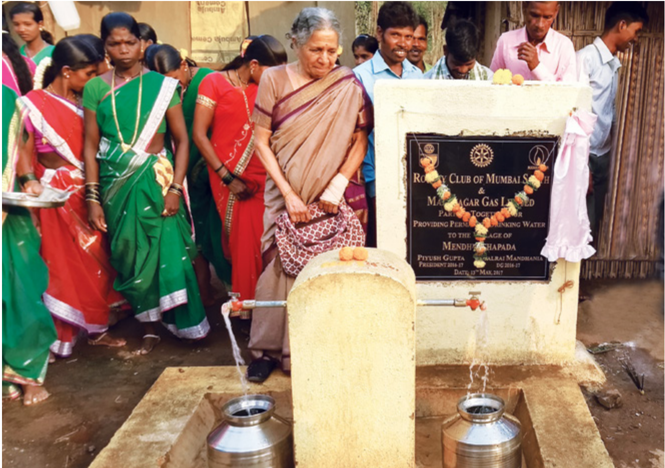
Safe Drinking Water Facility installed in Village Mendhyachapada under Naal Paani Yojana.
